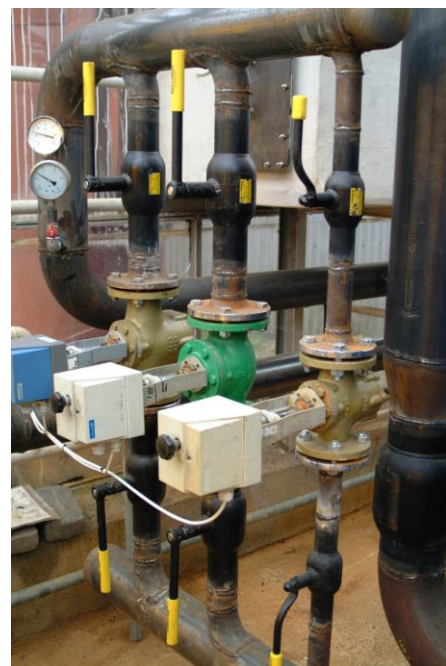
Figure 2 Valve actuator positioned on the floor
